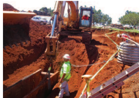
Grade checker Peter Morishige demonstrates the use of horizontal restraint system at sewer line excavation as Lee Iboshi (excavator operator) completes setting a trench shield
