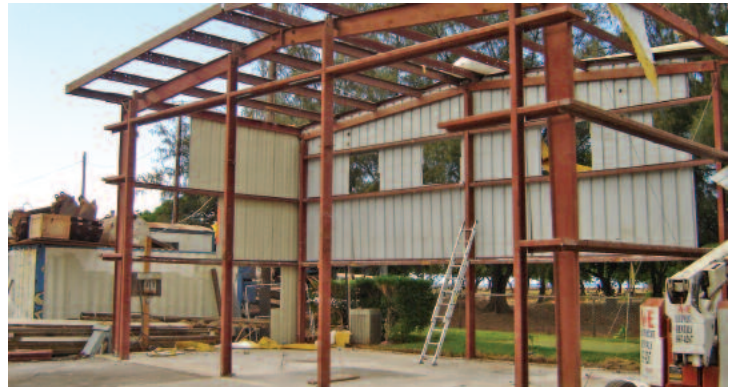
Disassembling Sand Island building for shipment to Hilo as new operations building
