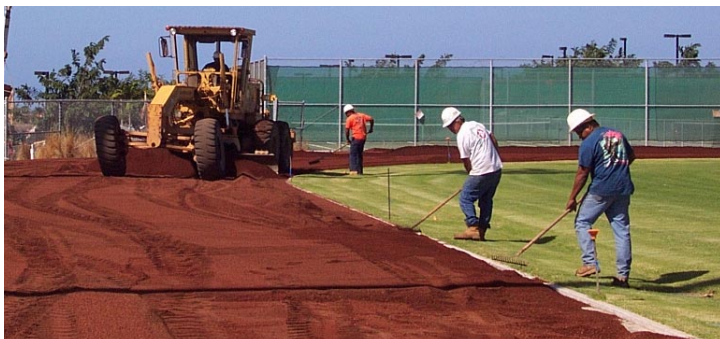
Finishing off the cinder track surface at Kealakehe High School with Dick Pacific Construction.
