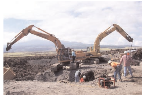
20 -inch double irrigation tie-in at Hualalai Clubhouse Loop Road with Kip, Jordan Sr., Derrick, Elvis, Byron, Camillo, Irving, Tommy, Cheston and Kubo.
