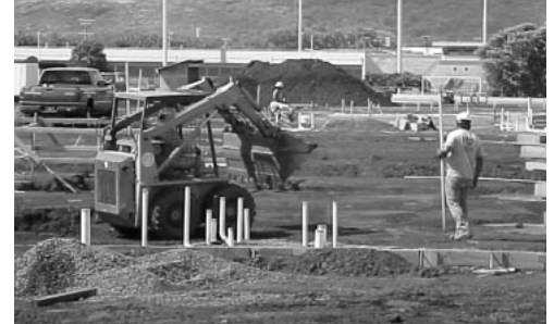
Kauai Police Station with Shioi Construction – Kip Furugen and Byron Ariola Kauai
